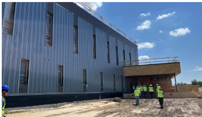
Figure 1: Construction underway of the new State Emergency Operations Center (SEOC). Photo credit: DPS
